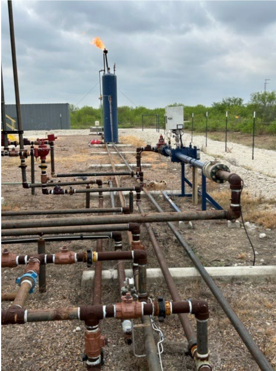
Flaring and pipe infrastructure at Cooke No. 7.
