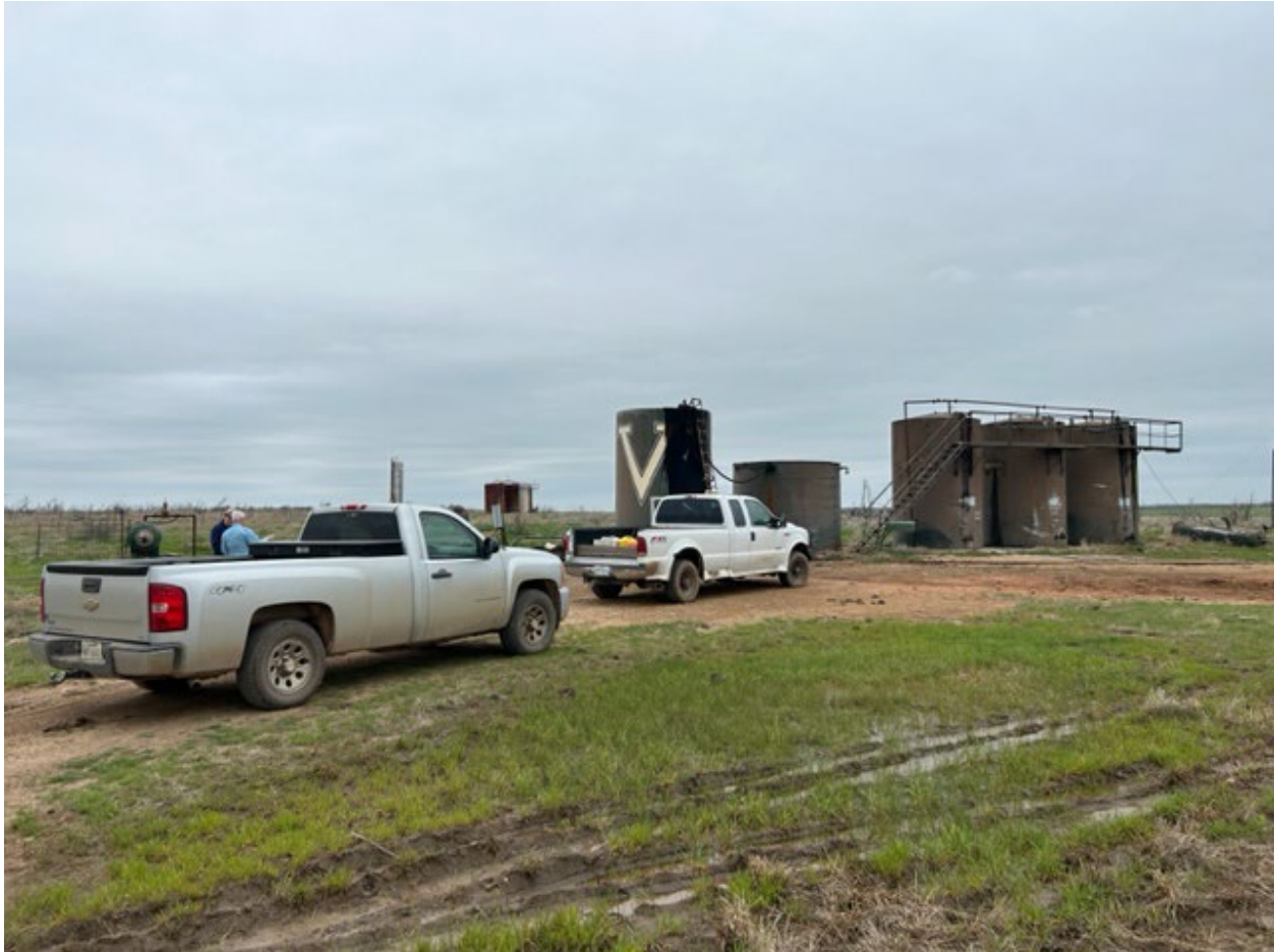
Kalkee's in place TCSL oil gathering and water dispersing equipment. April 2023.
